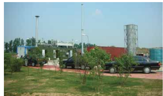
Figure 3.62 Central Electricity Generation Facility and Flare for Landfill Gas, Tianjin, China
